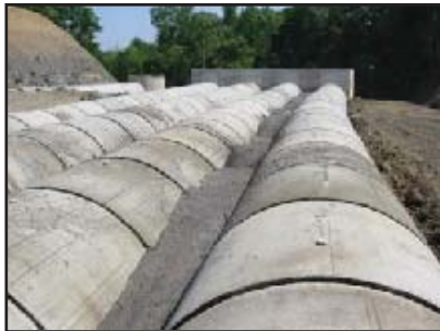
Flowable fill used as bedding for large concrete pipes. Foundry sand was used as fine aggregate in this flowable fill.
